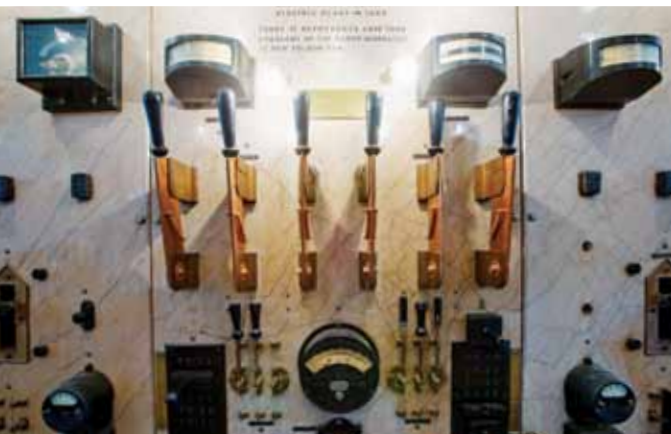
Insulating marble switchboard
