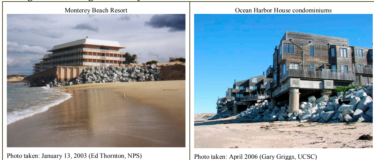
Figure 6. Armoring at Monterey Beach Resort and Ocean Harbor House Condominiums
