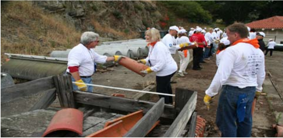
Above: Volunteers helped preserve and protect historic roof tiles by moving them to safekeeping in storage containers.
